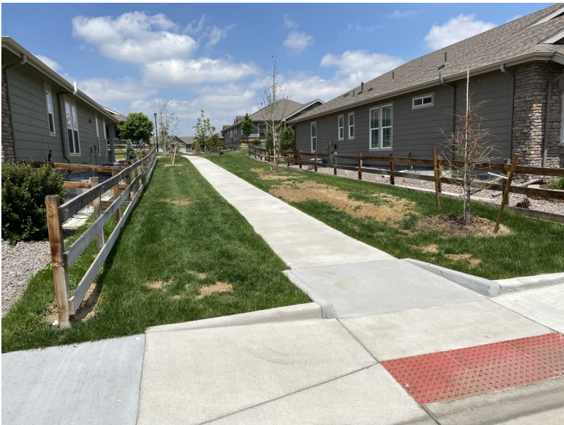
3. Remove dead sod. Fix grade so water does not pool here. Install new sod.
